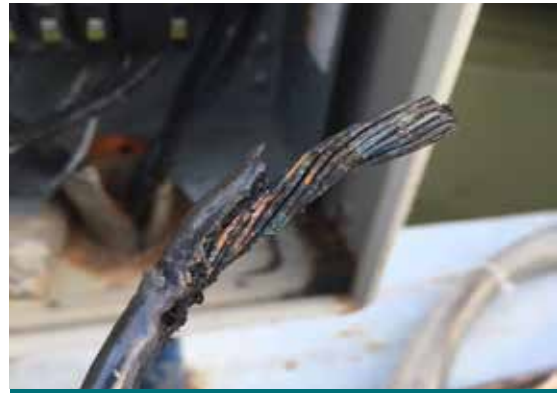
Frayed dock power box wiring
